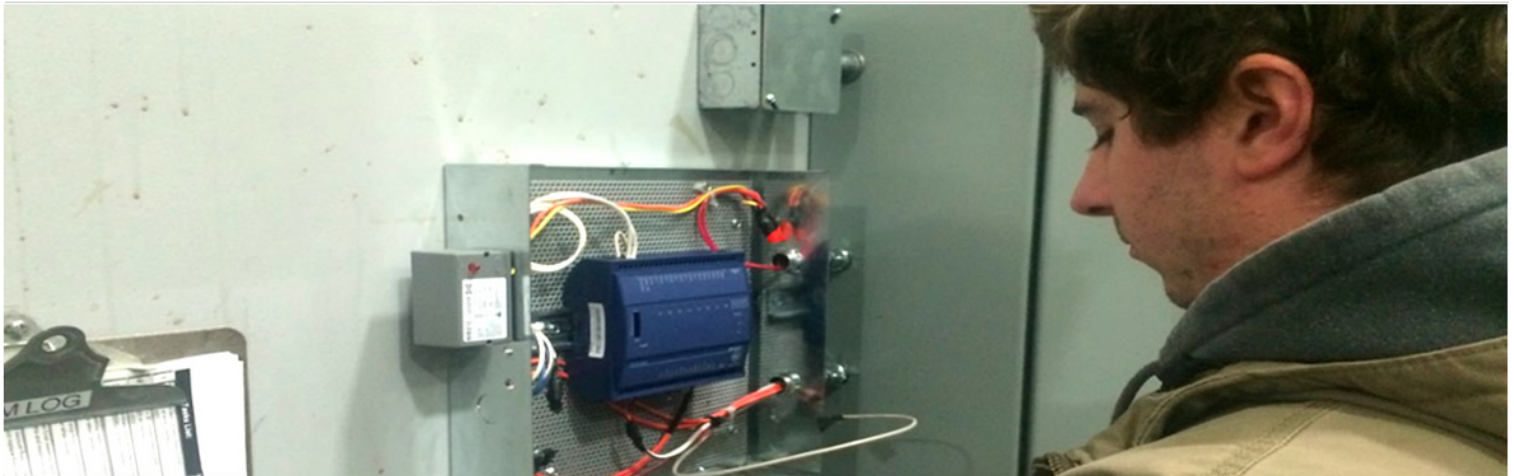
HEAT RECOVERY EQUIPMENT BEING CONNECTED TO AN EMS FOR MONITORING
