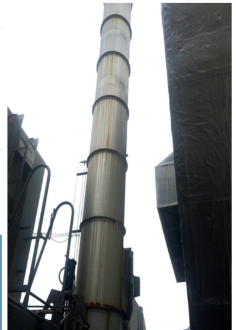
OXIDIZER EXHAUST WITH HEAT RECOVERY
