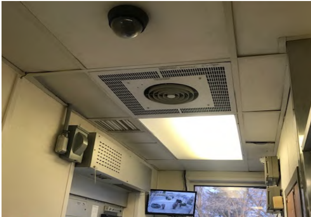
Uncontrolled electric heat now part of the automation
