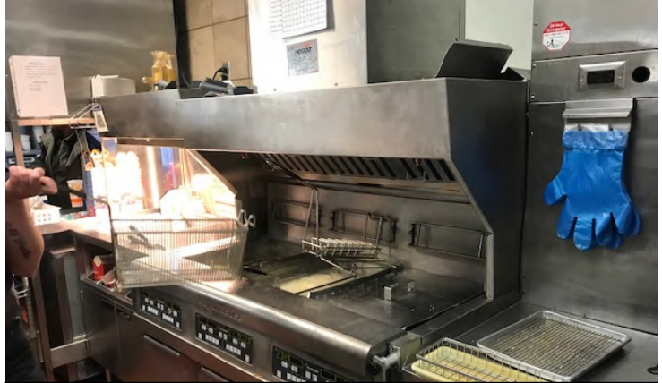
Kitchen area uses the RTU for MUA. Automation can control the building as a whole and balance the negative air
