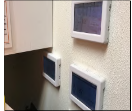
Each zone is now easily monitored and controlled remotely.
